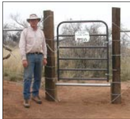
Laddie Cox with the help of San Pedro Hiking Club members Bill John, Ed Cleveland, Bob Powell, Jim Austin, Chuck Smallhouse, Hank Seane, and Ray Laase, recently installed a new gate on the AZT on the south end of Oracle State Park.
