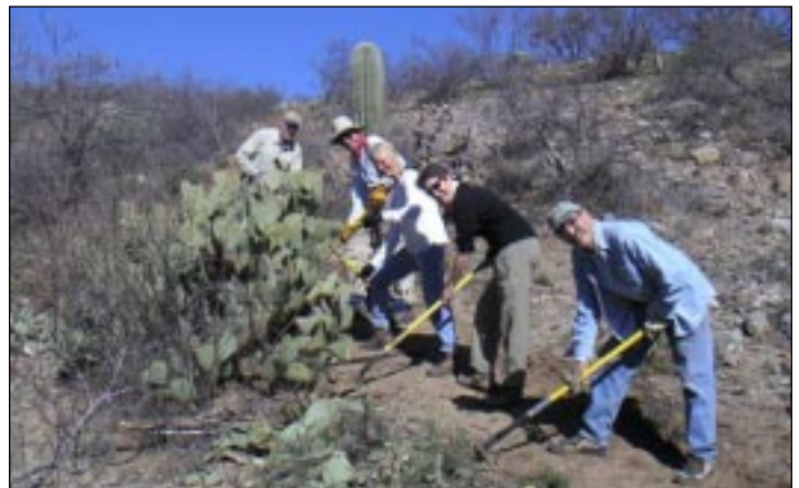
Group working on the Tucson/Black Hills section in late February, 2004. John Rendall recruited 5 volunteers for a session where they totally re-worked/re-built a portion of a switchback that had washed out with the summer rains. The volunteers are-- ( L to R) Jon Chase, Wayne Kennedy, Kathy Gish, Gwen Rendall, Jim Strickler. John took the photo!
