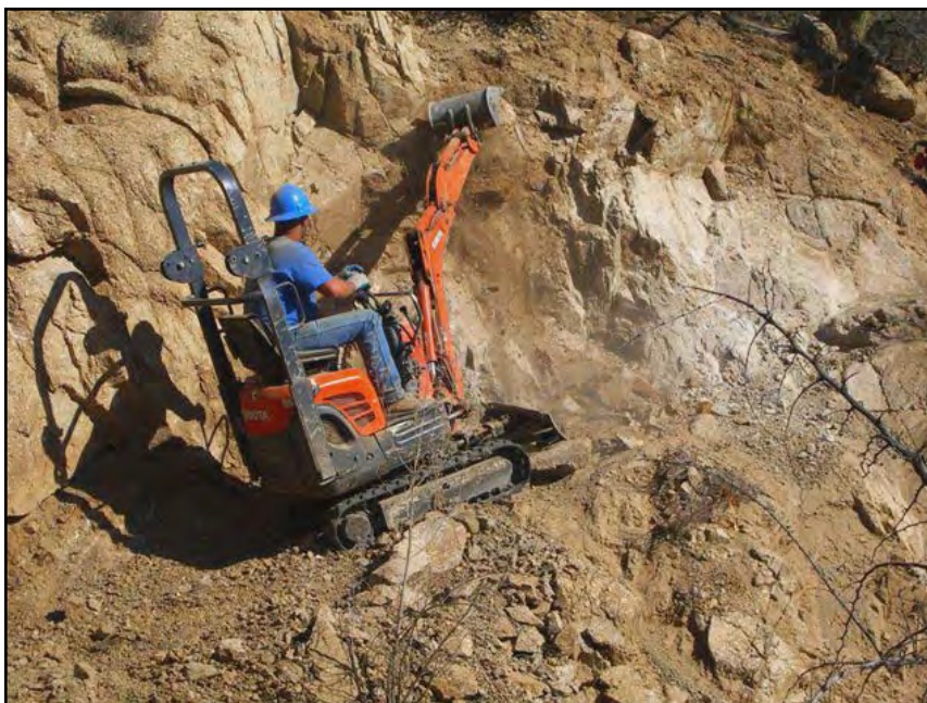
Mechanical trail machine makes progress on a rocky section in the White Canyon segment now under construction. Photo: Fred Gaudet
