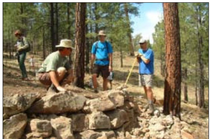
New switchback wall crew Anna, Paul Paonessa, Mike Faustich and Paul Meyer
