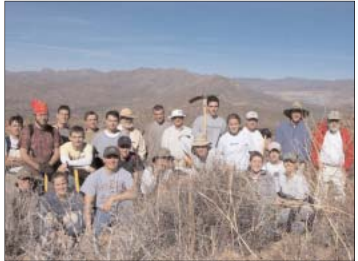
Segment Steward leader, Mike Luecker (in center, holding trail tool on his shoulder) and a large group of engineers with the American Society of Civil Engineers Phoenix Branch – Younger Member Group, joined with Crew Leader Merle Parmer, far right, to construct a section of the challenging Ripsey Segment of the Arizona Trail. This section of the Trail is approximately 2 miles south of the Florence-Kelvin highway, which parallels the Gila River in the central region of the state.
