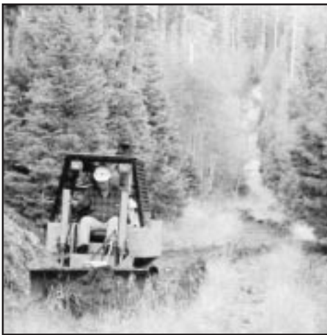
Chuck Horner operating the SWECO machine on new trail construction on the North Rim
