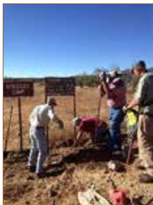
Digging out the old sign. No one expected to find a concrete base under it. Thank you Coronado NF for the jack hammer!
